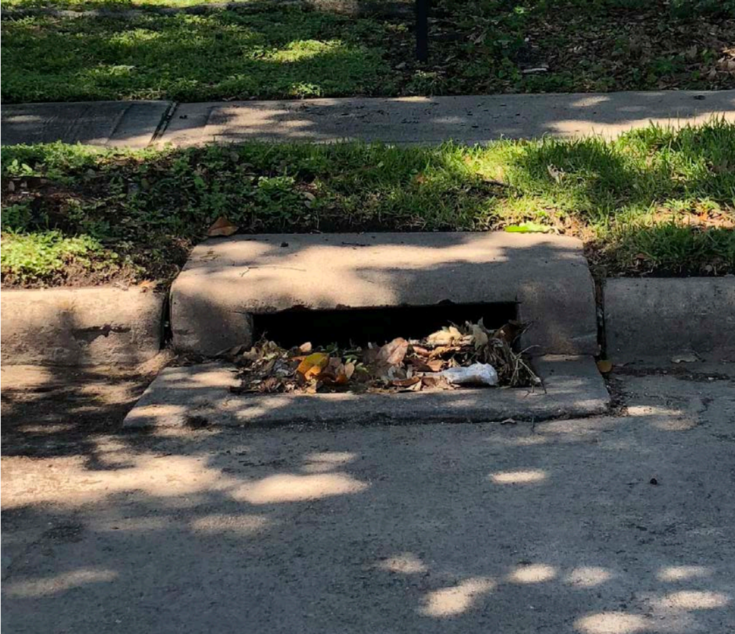
FIGURE 23. A BLOCKED STREET DRAIN HOUSTON. SOURCE: S.D. BRODY, TEXAS A&M.
